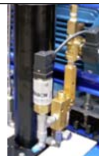
Filter Tower Pressure Bleed Valve
