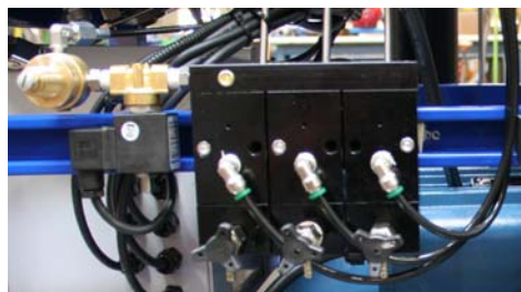
Auto Drain Valves with Manual Bleed Valves
