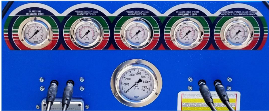
Figure 17. Oil, interstage, and final pressure gauges.
