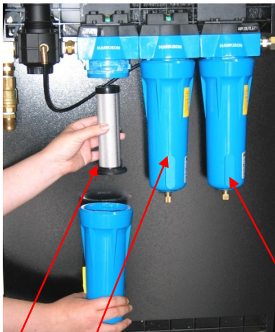
HF7 & HF5 Filters with Auto-Drain Floats & DP Indicators.
