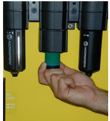
Changing LP Filtration Element
