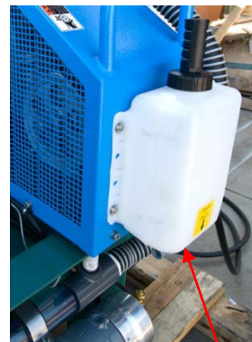
Condensate Drain Container. Check & Drain Weekly.
