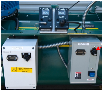
LP Feed Air Switch
