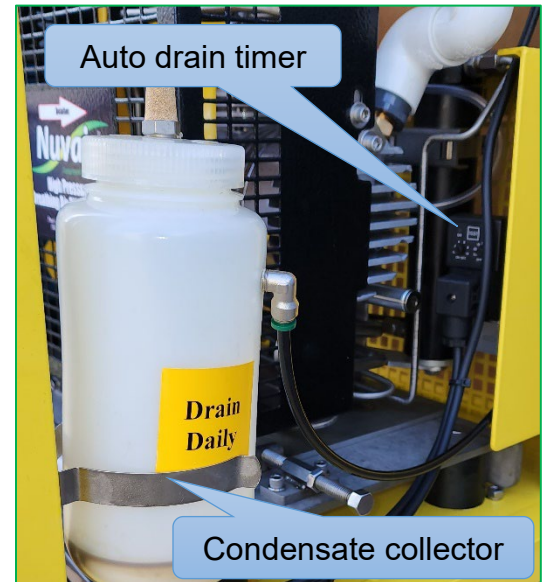
Figure 15. Condensate collector and auto drain timer.
