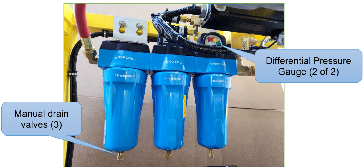
Figure 18. Inside frame view of LP filters.
