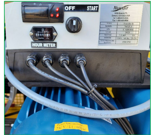
Figure 9. Electric Traveler power switch, heater temperature display, and hour meter.
