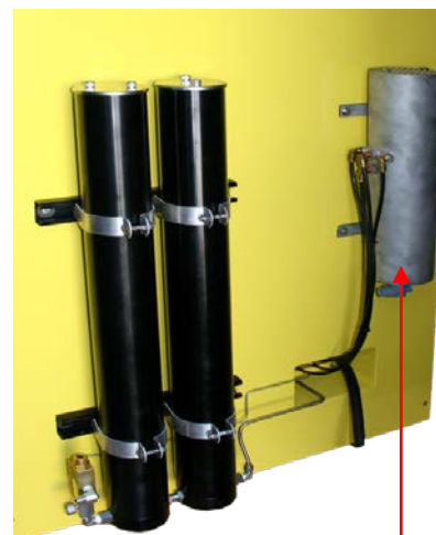
Condensate Drain Container. Check & Drain Weekly.
