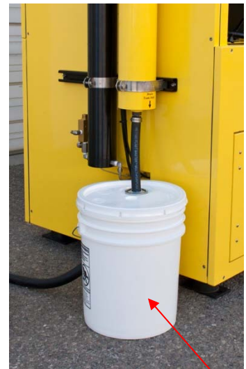
Condensate Drain Container. Check & Drain Weekly.
