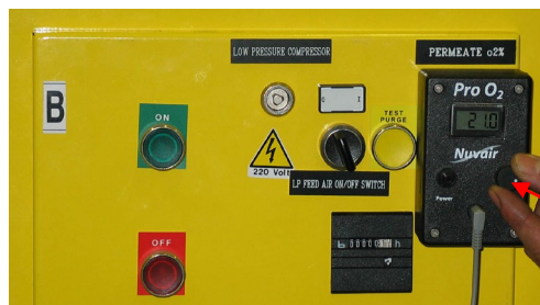
Permeate Oxygen Analyzer Provides Rough Reading
